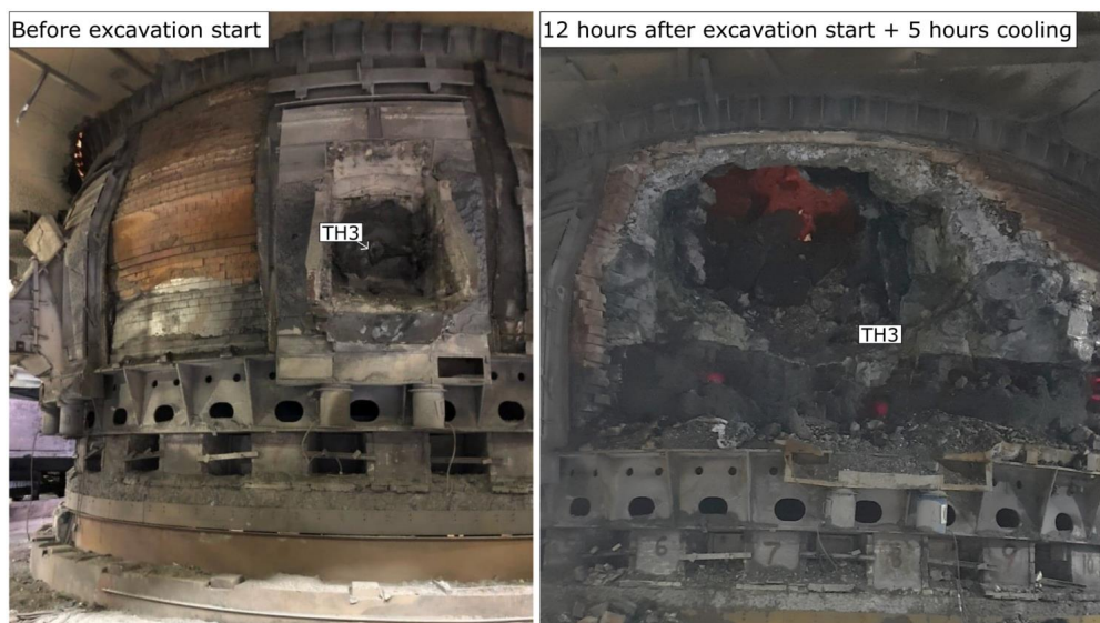
Figure 27 Photos of Furnace B taken right before excavation start and after the first 12 hours of excavating. The position of tap-hole 3 is marked in both images.
