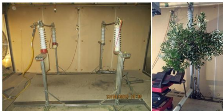
Fig.21 22 kV conductors and vegetation in contact
