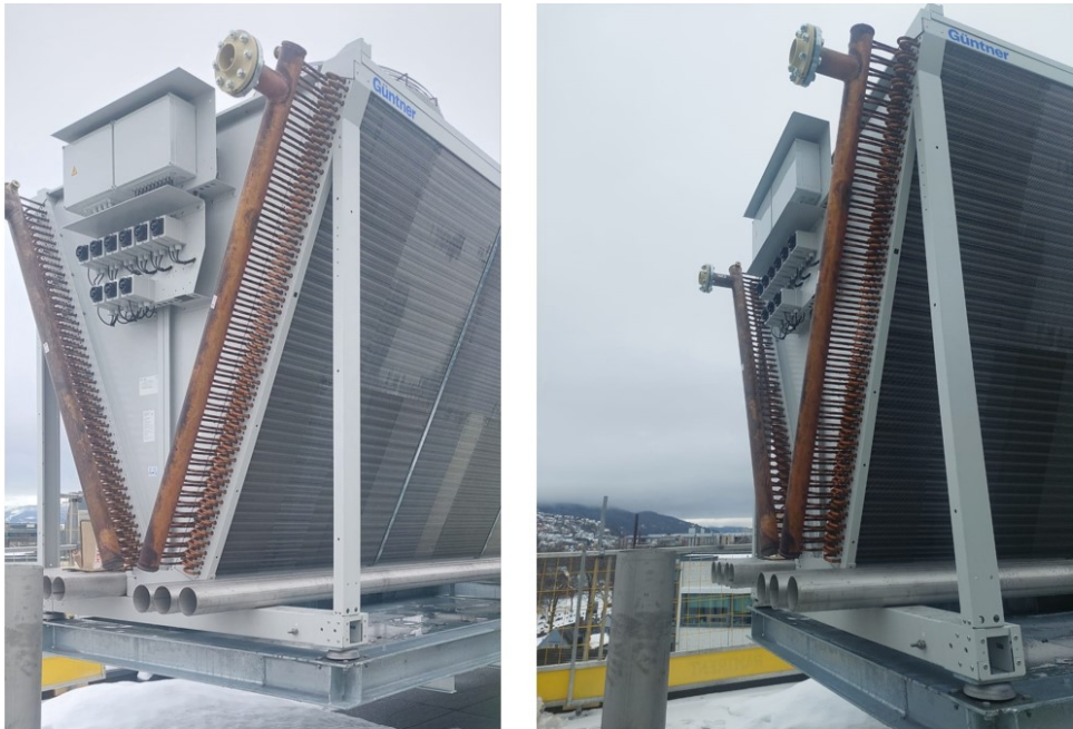
Figure 5.3: Pictures of the dry coolers of the system.
