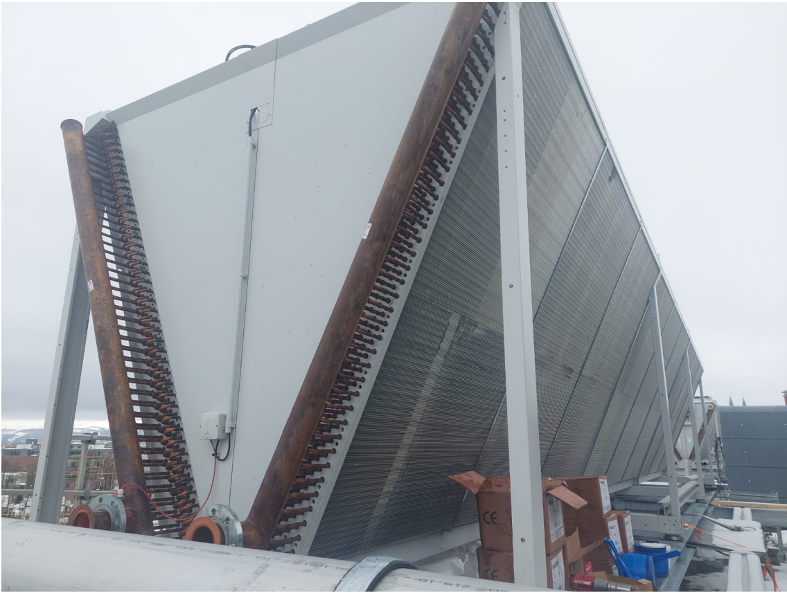
Figure B.2: Drycooler on the roof of AG5.
