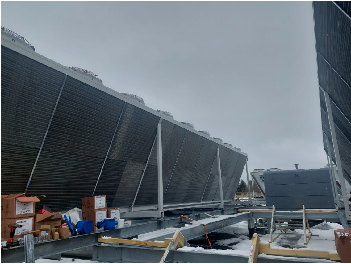
Figure B.4: Drycooler on the roof of AG5.
