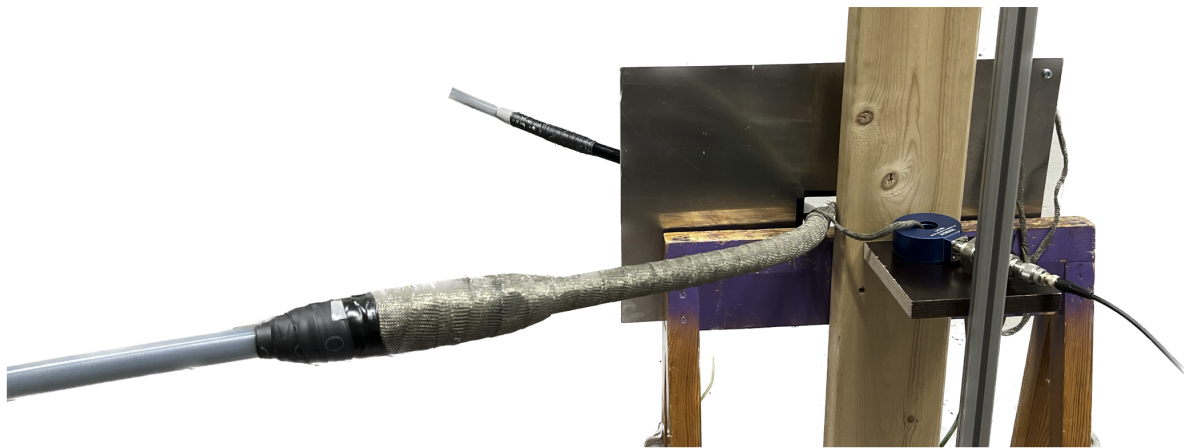
Figure 3.8: Terminated test object with applied termination tape and copper mesh. The copper mesh was applied over the termination tape and down the outer semi-conductor, to a total of 70 cm.
