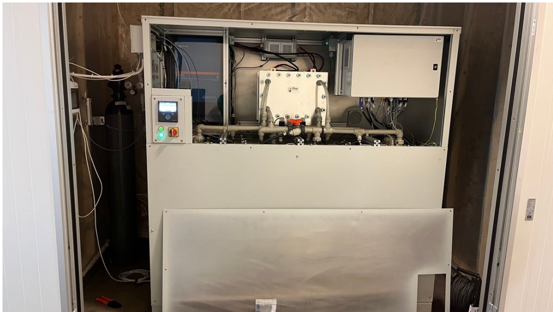
Figure 23: First flow battery installed in Norway-Lager 11, Sluppen (Author owns)
