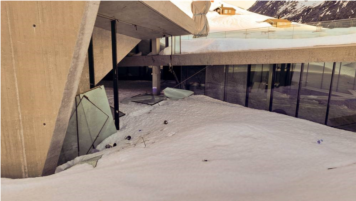
Figure 4-8. Broken windows and snow filling the visitors center, April 2022. Photo taken by Dag Christian Ugseth (Bjerknes and Sørensen, 2022).
