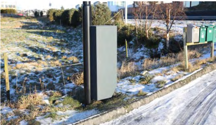
ELECTRIC CAR BATTERY: This box contains both measuring devices and a used electric car battery.
