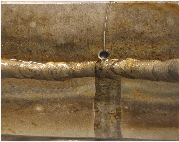
(a) Bad Weld Inside.
