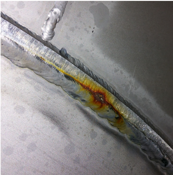
(a) Weld pitting at Mowi Ulvan
