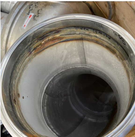
(c) Internal weld corrosion at InnovaNor
