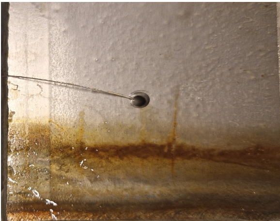
(c) Pitted Weld Inside.
