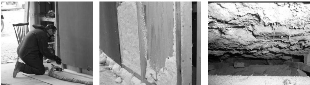
Figure 18 Example of cavity insulation of an 18th century house in Scotland. (Taken from Visual documentation process of historic building refurbishment "Improving energy efficiency by insulating wall cavity")
