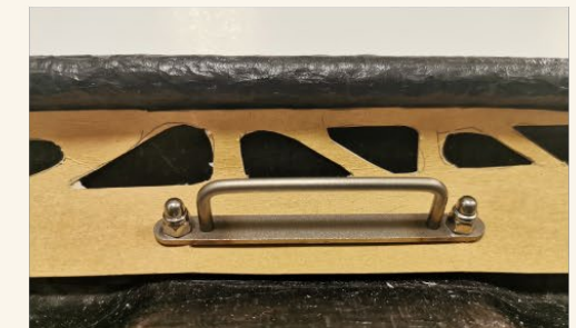
Figure 104. Illustration and measurement of available room for a plate beneath the existing brackets.
