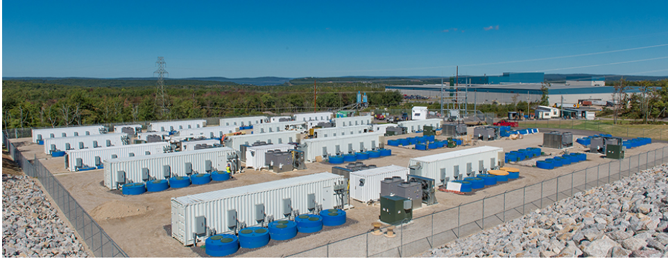
Figure 1.4: Beacon Power's 20 MW plant in Stephentown, New York [42].
