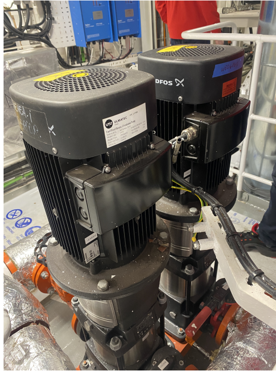
Figure 7.3: Main pumps connected in parallel on another SOV
