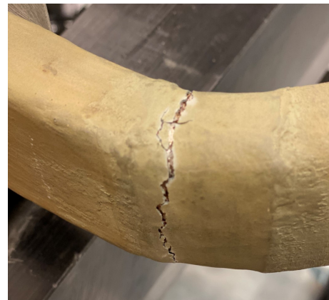
Fig. 6 – Crack in end-winding.
