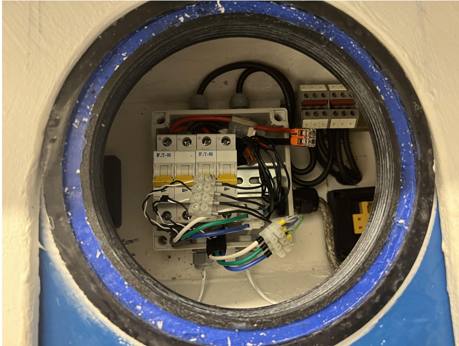
Figure 4.7: The junction box inside the hull (before mounting relays)
