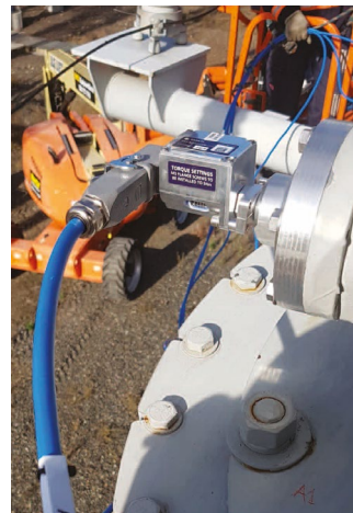
Figure 2. Bushing tap adaptor for Partial Discharge and bushing monitoring
