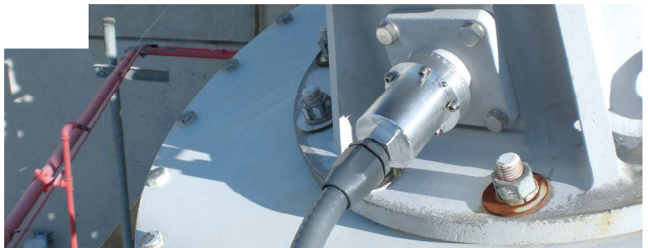
Figure 2. When installing a bushing monitor, it is important to ensure a secured installation and uncompromised contact with the test tap
