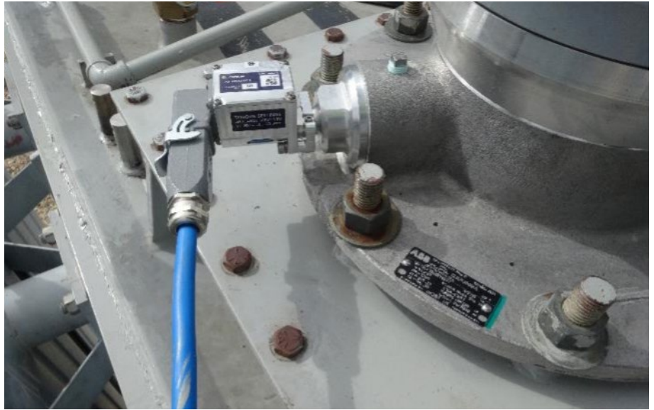
Figure 1: Kelvatek bushing sensor installed at the bushing test tap to detect both Partial Discharges and changes in Capacitance and Power Factor.
