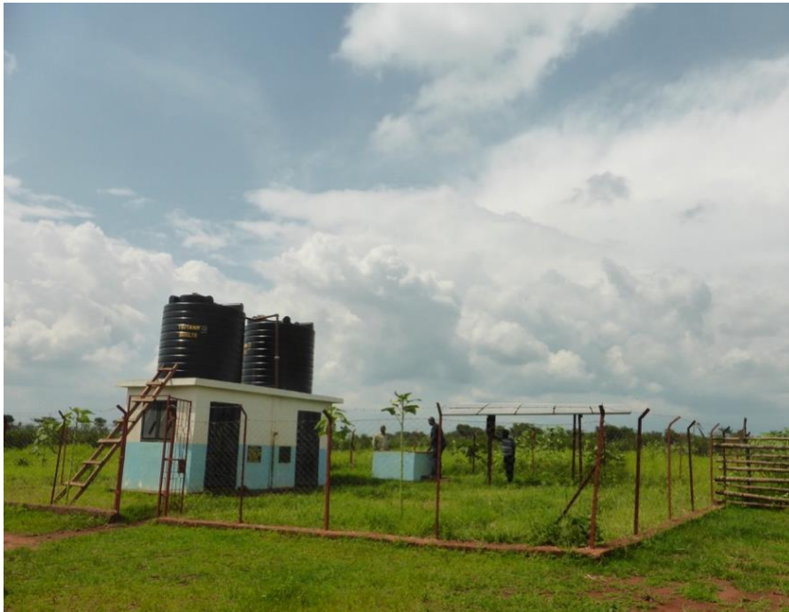
Figure 2.8: Solar powered pumping system in Endagaw Chini village with storage tanks, borehole (blue box in the middle) and solar panels.
