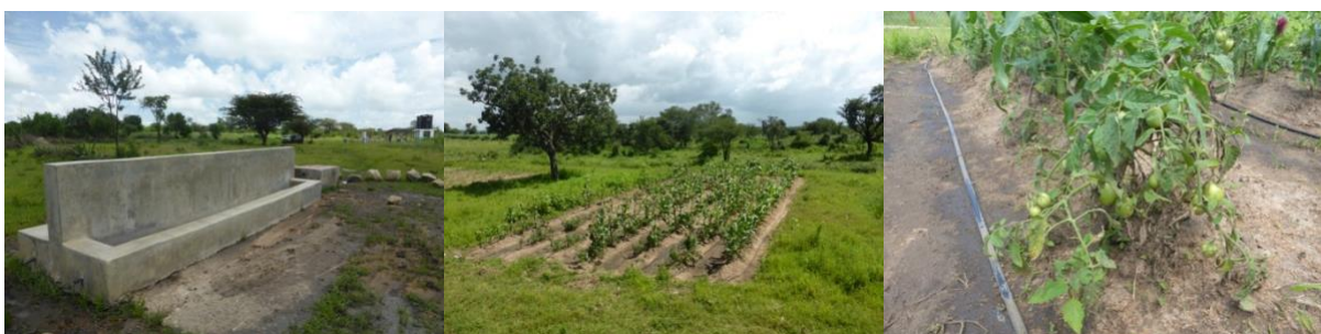
Figure 1.1: MUS-system installed by the NCA and 4CCP with cattle trough (left) and veggie-garden (middle and right) directly connected to the solar powered pumping systems.
