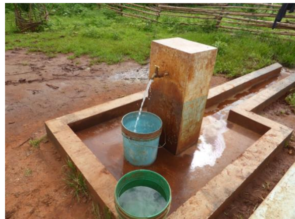
Figure 2.10: Water tap connected to the solar powered pumping system in Endagaw Chini.
