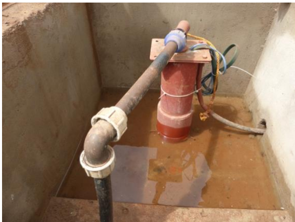
Figure 2.9: Borehole top of a solar powered pumping system.
