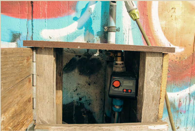
Automatic watering system set up
