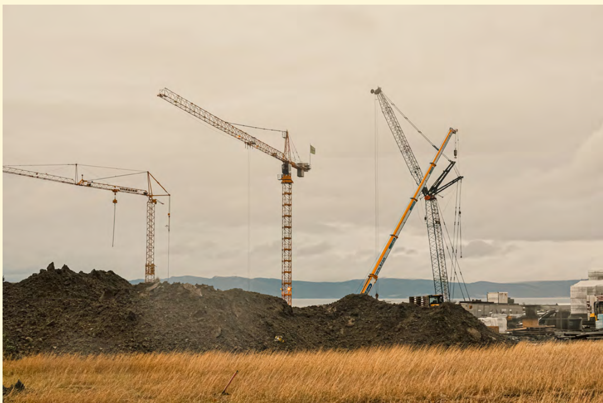
The heaps of soil is a manifestation of the priorities of the economy. Strinda Hageby
