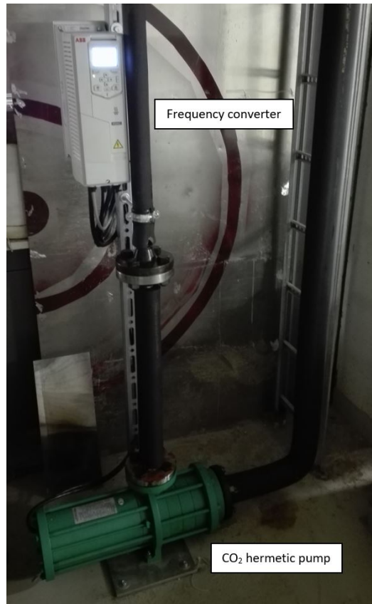
Figure 3.3: Hermetic CO 2 refrigerant pump with frequency control, supplying refrigerant circulation to the CTES unit.
