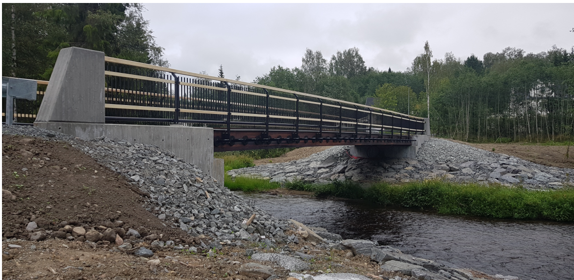
Figure 5.1: Photograph of the bridge analyzed in Raufoss. The picture was taken by Petter Juell Nåvik.
