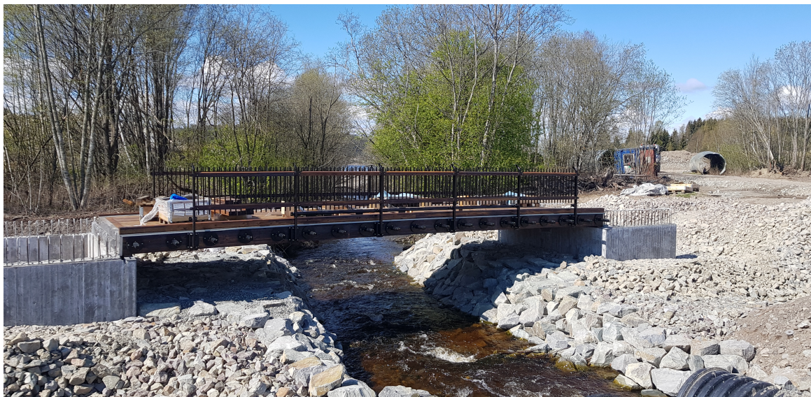
Figure 5.2: Photograph of the bridge analyzed in Brumuddal. The picture was taken by Petter Juell N avik.
