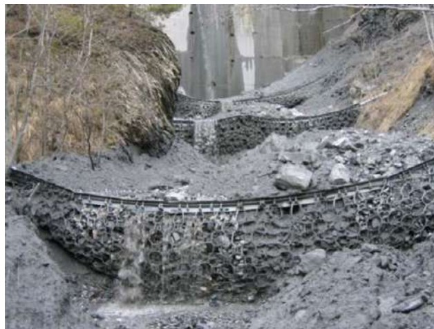
Figure 6.15: Three multilevel debris flow barriers in Merdenson, Valais, Switzerland. Similar barriers are planned used as mitigation measures against slush flows in Longyearbyen, Svalbard. Source: Wendeler [95].
