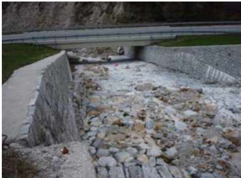
Figure 6.13: Bridge over slush flow drainage road with channelising walls on each side. Photo: Harald Norem. Source: Vegdirektoratet [32].
