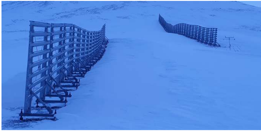
Figure 6.11: Snowdrift fences with horizontal steel boarding in Longyearbyen, Svalbard. Photo: Haldis Døvre Kalland.
