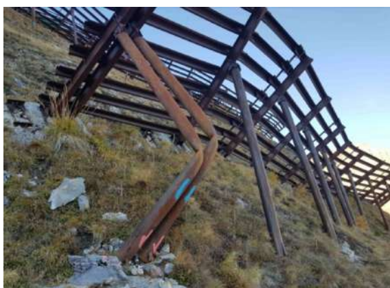
Figure 3.1: Snow supporting structure with buckled supports at the end of the structure line, Valais, Switzerland. Source: Margreth [25]. Photo: Nivalp SA (2018).
