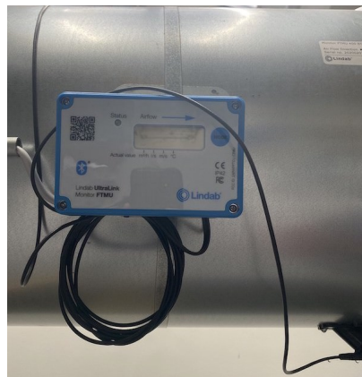
Figure 3.19: Lindab UltraLink to measure the total ventilation airflow rate.
