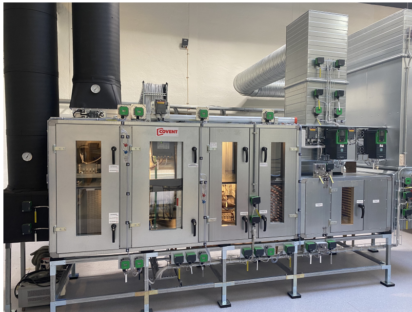
Figure 3.3: Air handling unit from Covent at the HVAC-lab at Gløshaugen, NTNU.
