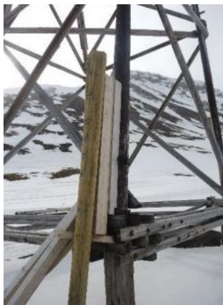
Figure 2.6: Picture of a bolt connection between a column and a supporting pile. Picture adapted from [7].
