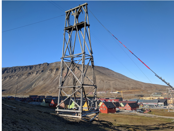
Figure 2.5: Picture of the cableway post in the alpine slope of Longyearbyen, marked with B in figure 2.3. The photo is taken after the rehabilitation. Photo taken by Author.
