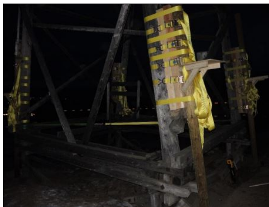
Figure 2.7: The picture shows how the new solution with 8 straps as connection between the columns and the supporting piles were used. Picture adapted from [7].
