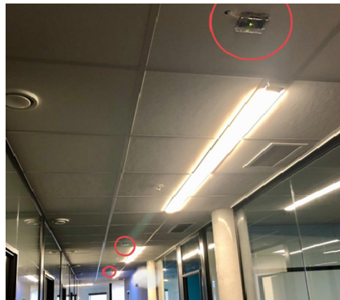
Figure 4.4: POE dev boards placement in the office hallway. Source: Private photo
