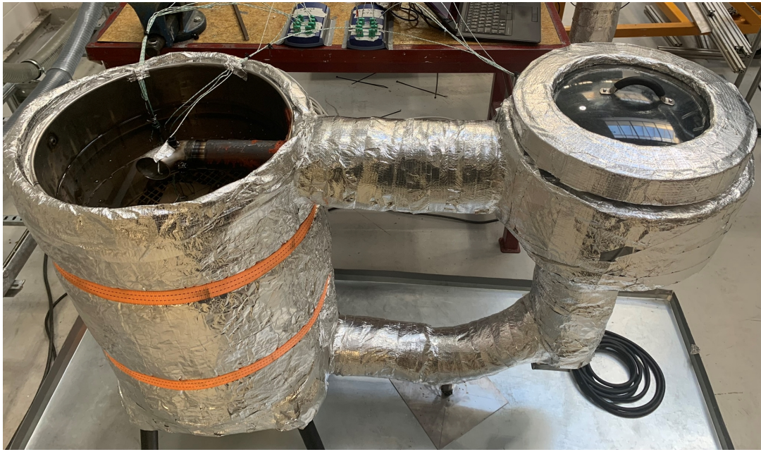
Figure 3.13: Completed Dual Tank System with insulation without the barrel lid
