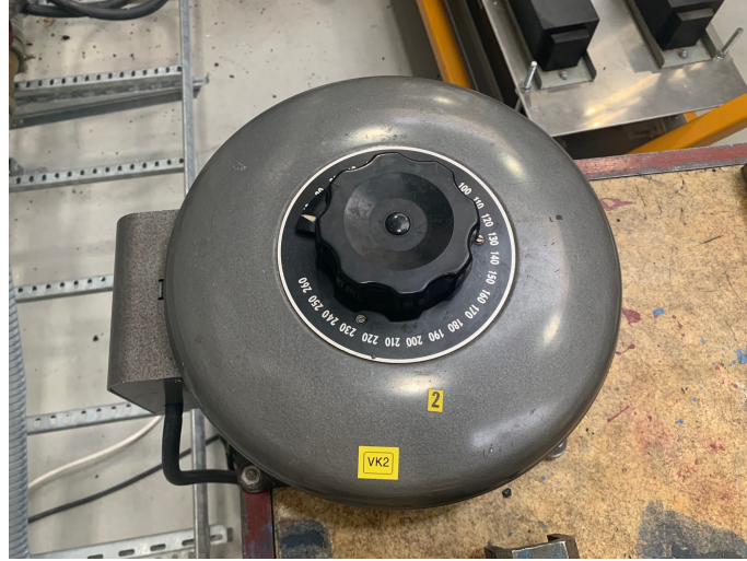
Figure 4.2: Variable voltage transformer used for testing
