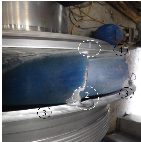
Figure 2. Erosion at different locations of runner inlet; Locations 1-2 refer to the region affected by the leakage flow from GV's clearance gap, and locations 3-4 are regions affected due to leakage flow from sidewall gaps.
