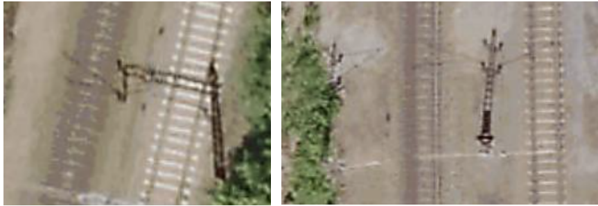
(a) EH-MAS-023298 mast at Sjøberg station. One pole supplies both tracks with cantilever. (b) EH-MAS-023371 (left) and EH-MAS-023370 (right) masts at Melhus station. Two masts supply the right track line with cantilever.
