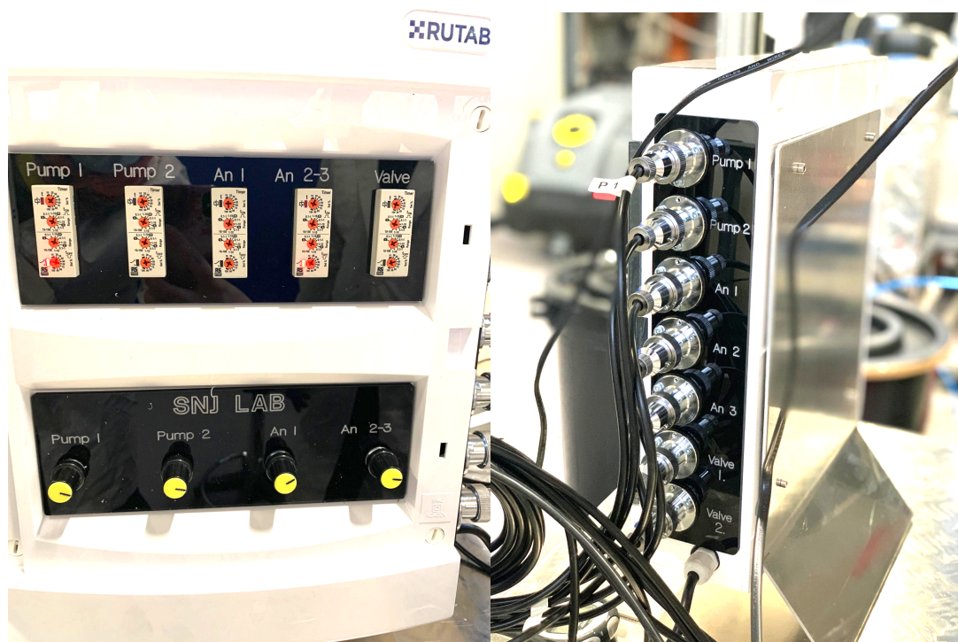
Figure 13: Control panel for the lab - scaled pilot.
