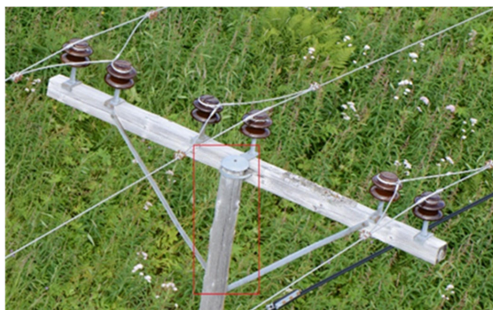
Figure 7. Wooden pole where a crack has been localized on the mast (see rectangle).
