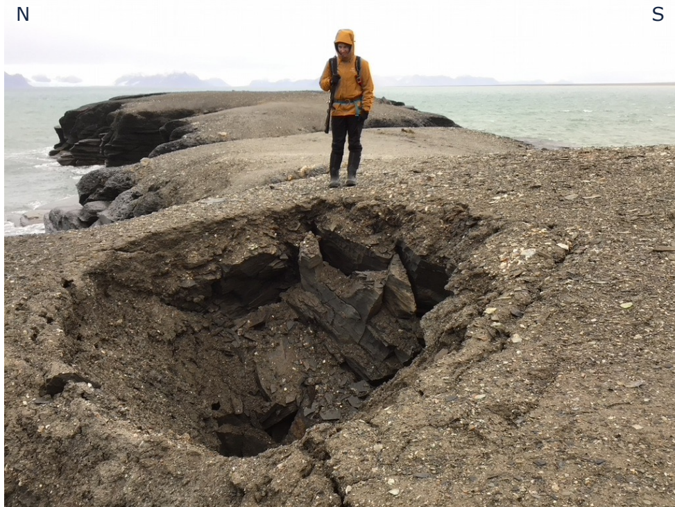
Figure 34 Ground collapse. Reinhardpynten is behind the person. Location of photo is 78°33'31.59"N, 011°18'7.73"E.
