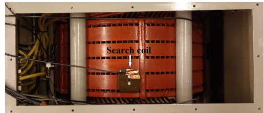
Fig. 10. Location of a noninvasive search coil sensor to capture the stray magnetic field installed on the back side of the stator yoke.
