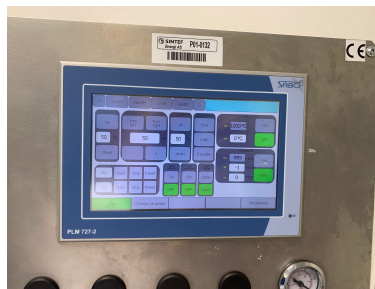
Figure A.8: Control board.
