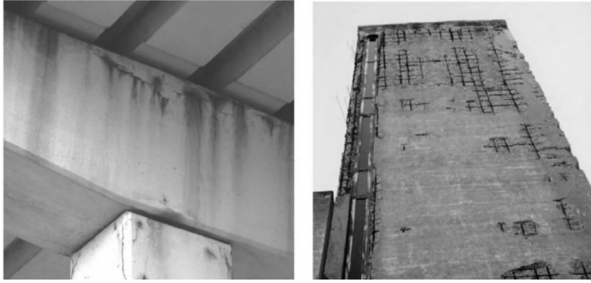
Figure 9: Examples of consequences of corrosion of steel in concrete (Bertolini et al. 2013).
