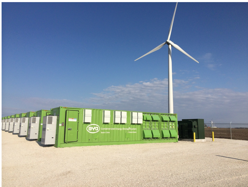
Figure 6.1: 31.5 MW Grand Ridge Storage Facility located in Illinois, USA [78].
