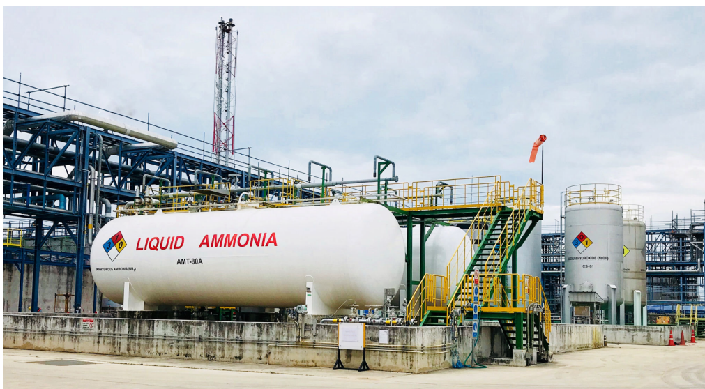
Figure 2.16: Refrigerated liquid ammonia storage tanks [86]
