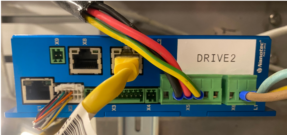
Figure 74: Nanotec N5-2-1 motor controller electrical wiring
