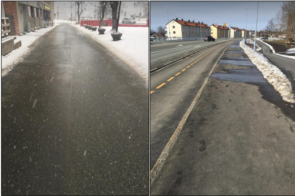
Figure 1 Surface conditions categorized as "Asphalt"
