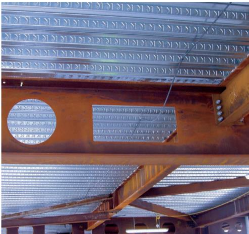
Figure 1: Example of unstiffened rectangular and circular openings in the web of a steel beam [1].
