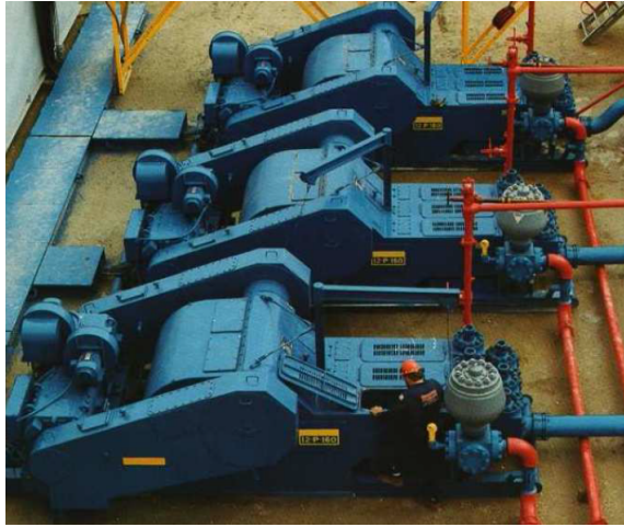
Figure 1: National Oilwell Varco (NOV) Triplex mud pumps, type 12P-160
