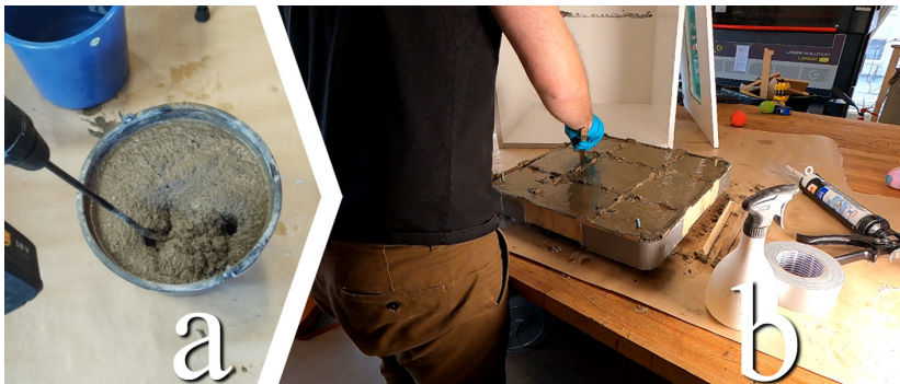
Fig. 23. a) Mix concrete thoroughly in accordance with package. b) Pour concrete, distribute and pack it with a stick.
