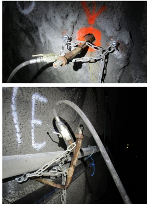
Fig. 8: Example of packer anchoring. Upper photograph showing how the packer rod is mechanically secured to the tunnel wall using expansion anchors and a chain. The lower photo shows how a packer rod was bent after a sudden packer release
