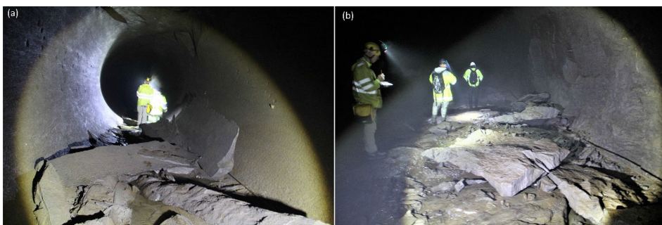
Fig. 16 Block falls registered in a hard crystalline rock (Trondhjemite) and b schistose phyllite during inspections of unlined pressure tunnel of a power plant in Norway
