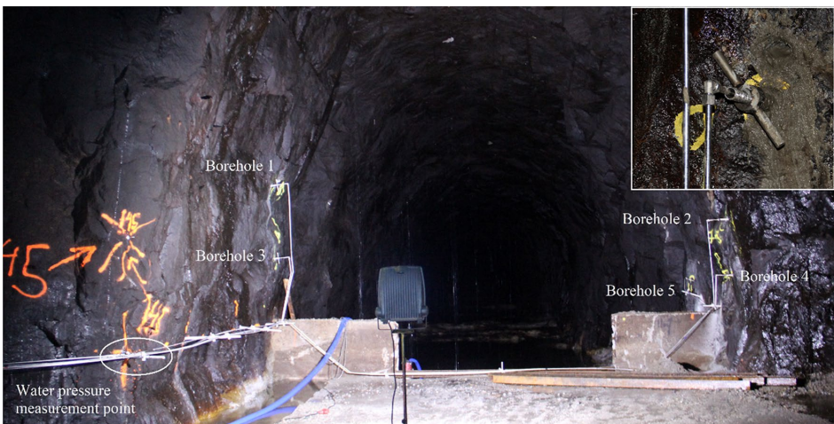
Fig. 8 Location of boreholes in the tunnel (looking upstream) and detail (top right corner)
