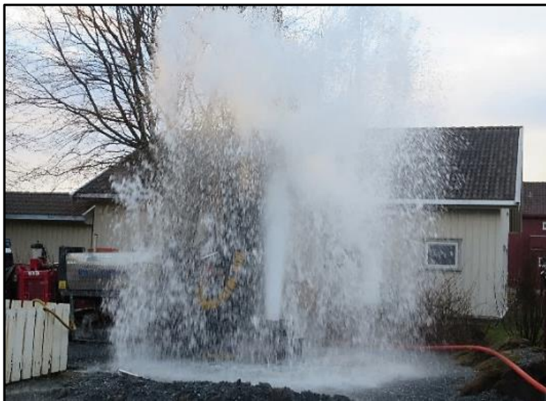
Figure 2-3 Periodic airlifting, shocking and flushing, of the groundwater well is crucial for developing a proper naturally developed well filters (Photo: Randi Kalskin Ramstad).
