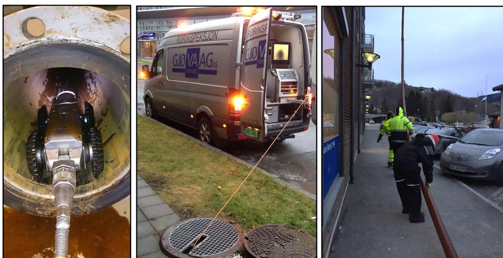
Figure 3-2 Video inspection of wells. (Left) The Supervision TM SVR 140/SVC100 pan and tilt video camera (Gjøvaag AS). (Middle) The camera is remotely controlled from the inspection vehicle (Gjøvaag AS). (Right) In this Melhus installation the pipe is 24 meters long and a large crane and several people had to help in order to lift it out of the well bore (Picture by Mari Helen Riise).
