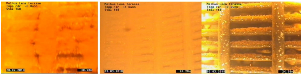
Figure 4: Picture at left: The well screen is tight before rehabilitation in February 2018 when the water was flowing over. The blurry picture is caused by a thin film on the camera lens. Picture in the middle and at the right: Video inspection of the well screen after jet flushing with mixed results. The pictures are within 10 centimeters, and large parts of the screen is still clogged with precipitated iron oxides (middle), while the natural filter of sand and gravel can be seen in some parts (right picture)
