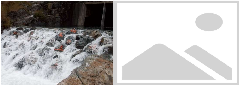
Figure 1. Dam crest exposed to overtopping, Photo: Leif Lia
