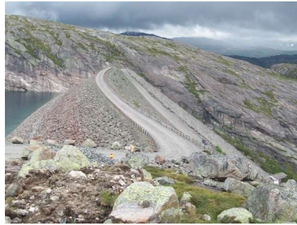
Figure 5. Dam crest with suitable freeboard and cover of core materials, Photo: Leif Lia
