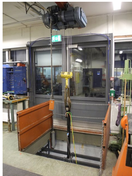
Figure 4.44. Crane used for lifting heavy equipment. Here with the actuator placed on the actuator frame.
