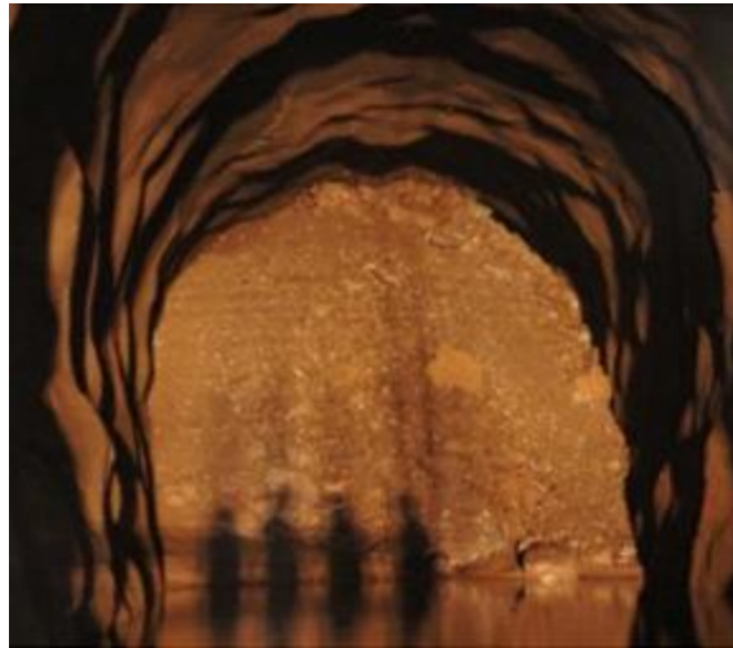
Figure 6.3: Weathered rock associated with the geological fault at the collapse location of La Higuera headrace tunnel (Brox, 2019)
