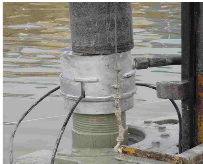
Figure 5.7: Modified grouting cap used to pump grout into the borehole in Dörverden.
