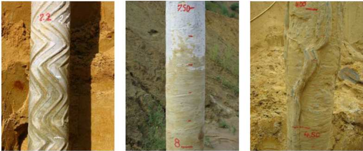
Figure 2.6: Excavated grout bodies from Tomboy and Huybrechts (2008): Cased drilling with internal flush (left), drilling with external flushing after primary grouting (centre) and after postgrouting (right).
