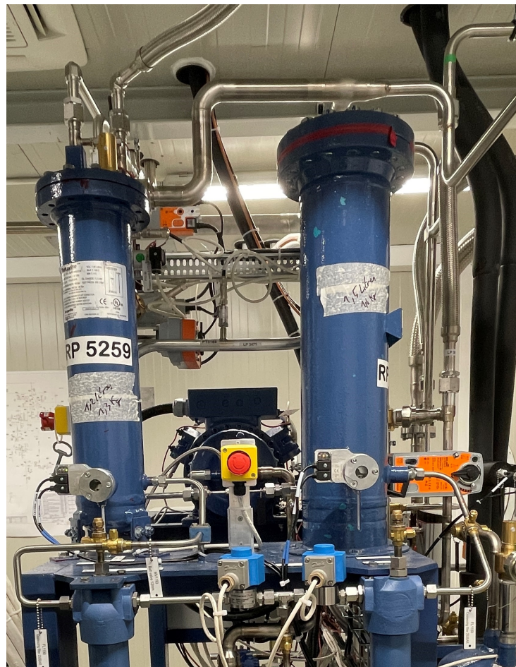
Figure 7. Coarse and fine oil separators installed in one of the compressor slices.
