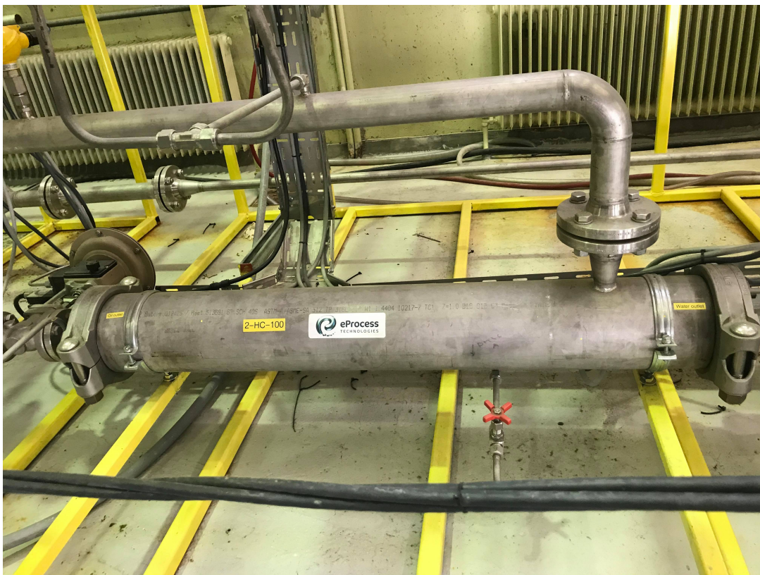
Figure 2.3: Photo of the hydrocyclone
