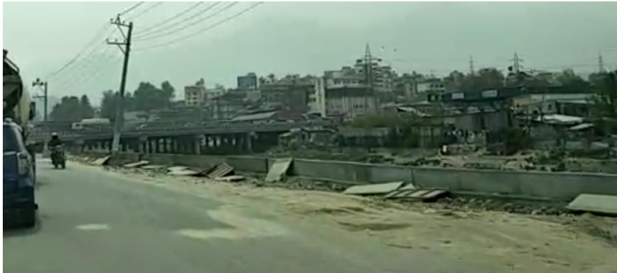
Figure 5-49/50/51 Ongoing construction moving towards the south boundary of the case study (taken from video captured by field assistants, 2021)
