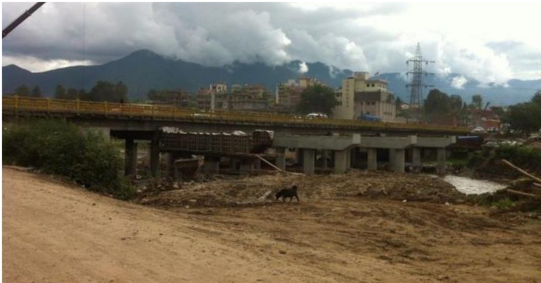
Figure 5-34 Structural expansion of the Balkhu bridge going on in 2015 (provided by Dr. Niva Baral)
