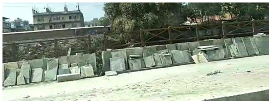
Figure 5-48 Footpath and wall construction within case study area (taken from video by author’s field assistant, 2021)
