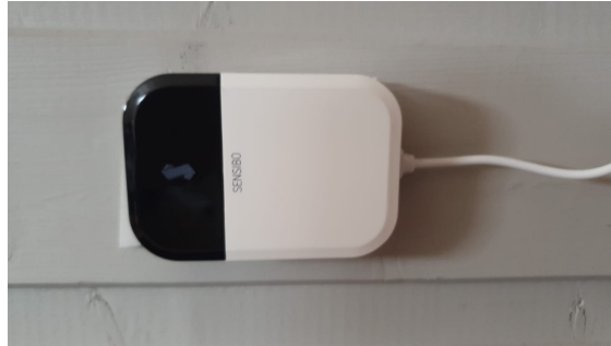
Figure 6.4: Photo of one of the Sensibo Sky devices on the wall of the house. There are four of these in the house, one for each heat pump.
